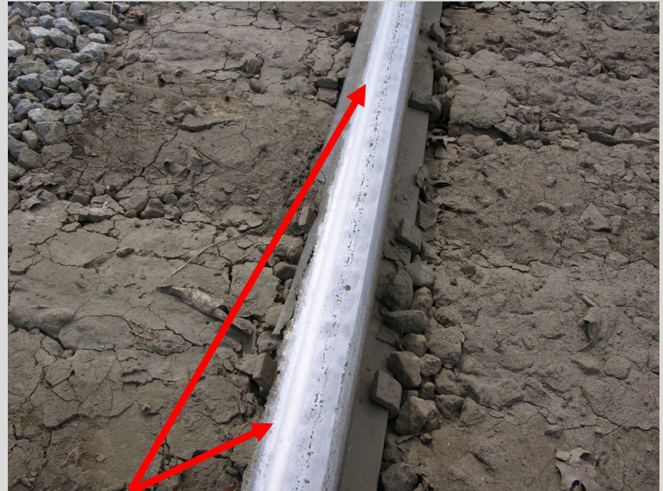
Evidence of false flange contact on field side of low rail another way of finding wide gage and broken spikes
